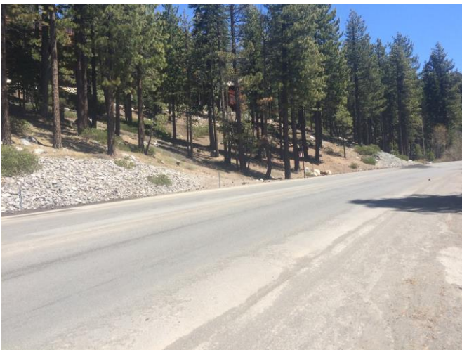
Figure 3: May 12, 2017 sediment on road.
