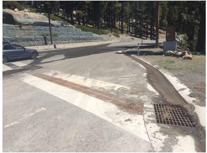
Figure 2: May 12, 2017 sediment on pullout and road. Snowmelt flowing into drop inlet.
