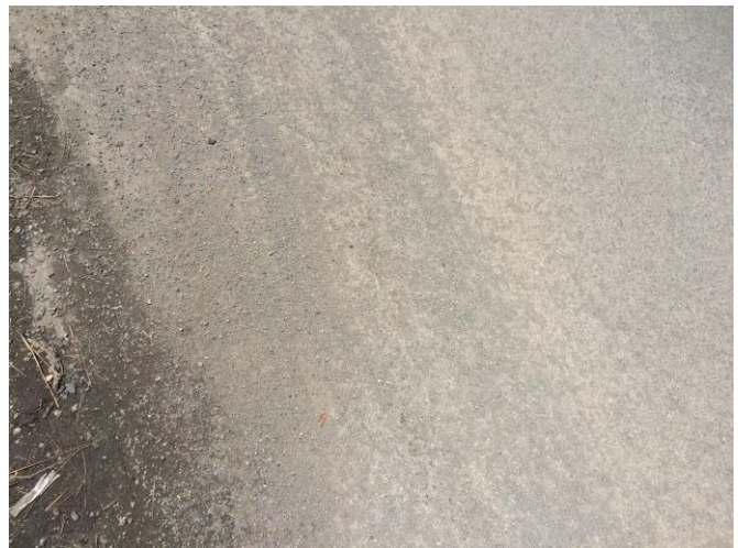
Figure 4: May 22, 2017 sediment on road.
