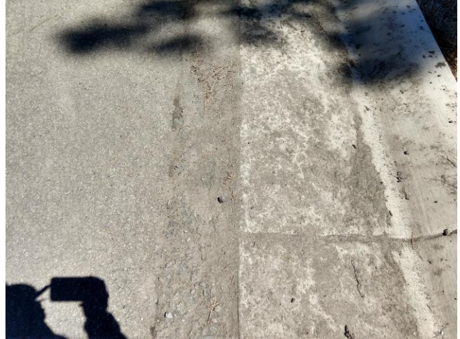
Figure 2: April 20, 2018 sediment on road.
