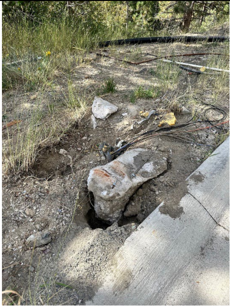
Figure 1 Jobbox holding equipment ripped off of base, tearing and exposing wires on September 15, 2023.
