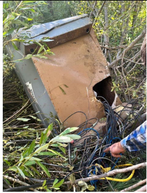
Figure 2 Jobbox housing sensitive monitoring equipment found a few hundred feet down the embankment on September 15, 2023.
