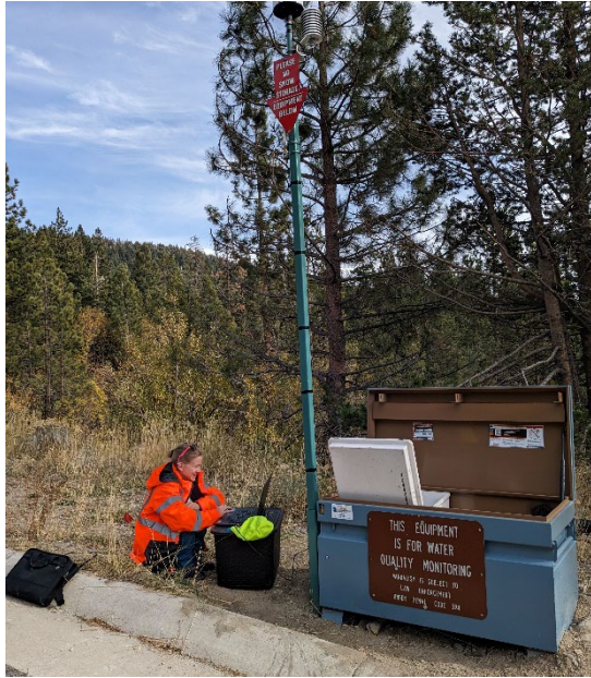
Figure 5 Troubleshooting and testing equipment on November 1, 2023.
