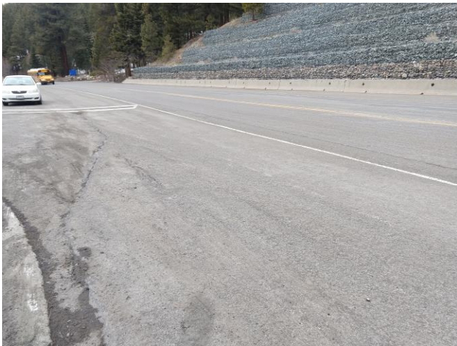
Figure 5: SR431 on March 17, 2021.
