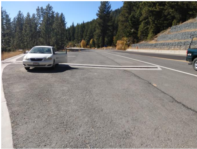
Figure 3: Light sediment on road October 25, 2019. Road RAM score of 2.2.
