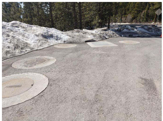
Figure 2: Berm on SR431 pullout on February 20, 2020. This berm did not inhibit access to the sites.
