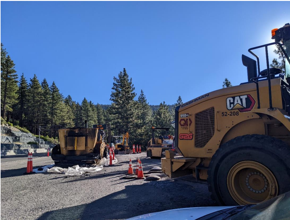
Figure 134 Construction activities at SR431 on September 29, 2022. A pressure transducer was severed during construction activities which caused a power short. Luckily only minimal damage occurred. It is crucial to communicate locations of monitoring equipment with construction staff to avoid damaging monitoring equipment.
