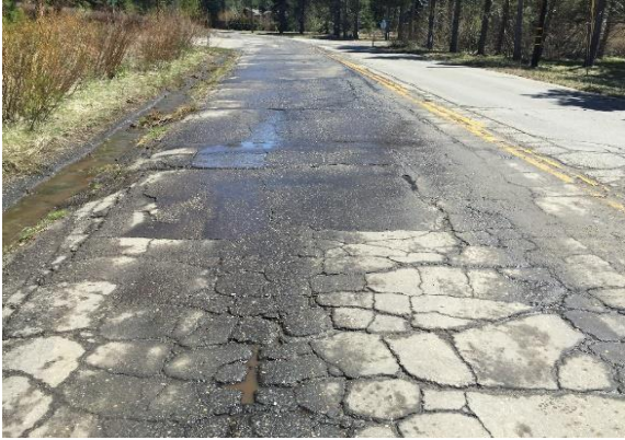
Figure 73 Elks Club Drive prior to repaving. (R Wigart)
