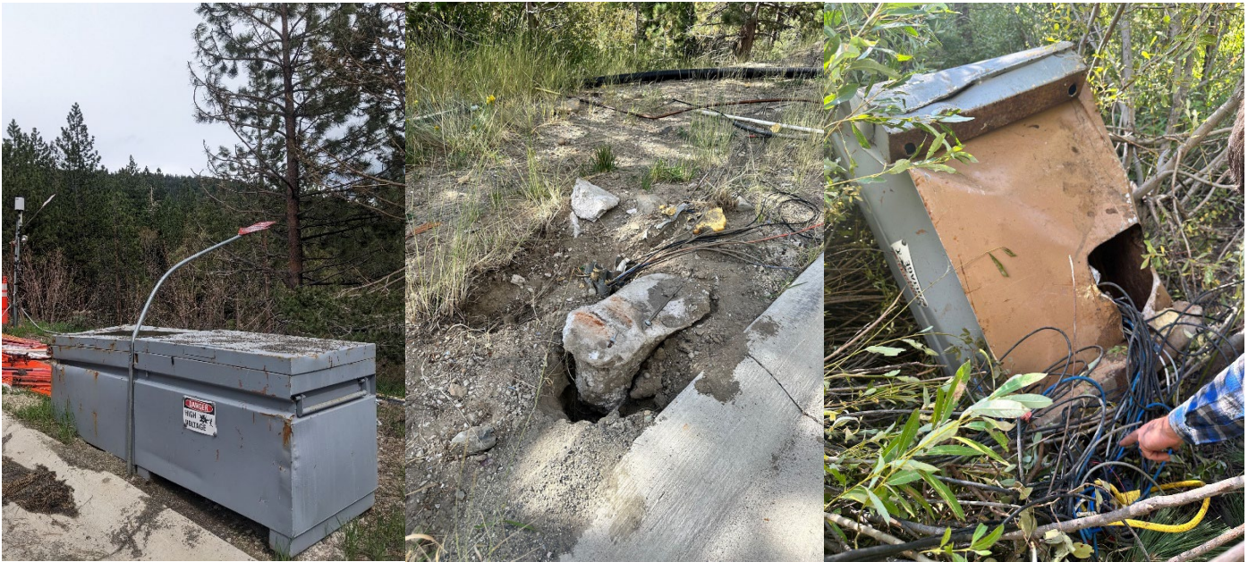
Figure 134 Boxes containing monitoring equipment at SR431 before the car accident on September 15, 2023 (first image), and after the car accident showing ripped cables where equipment boxes used to be (image 2) and box pushed down the embankment (image 3).
