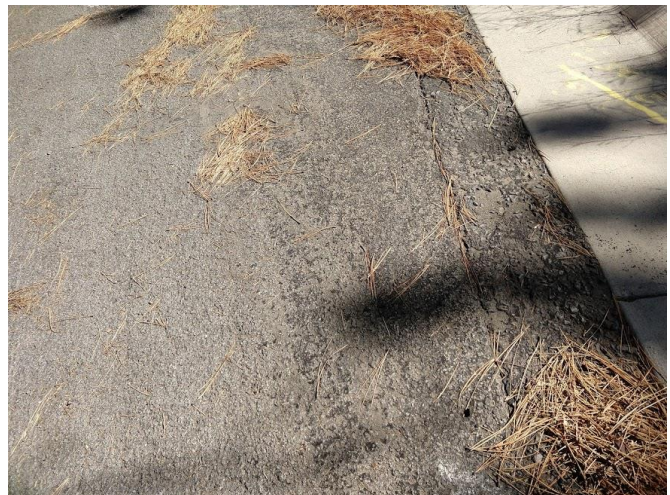
Figure 2: October 12, 2019 sediment on road.
