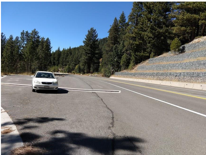
Figure 1: October 12, 2019 SR431 pullout.
