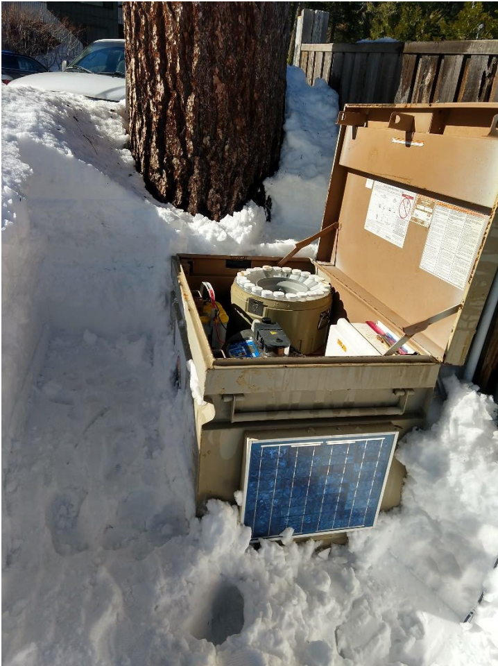
Figure 132 Tahoma on February 1, 2021. It is critical to stay on top of snow removal after snowfall events to maintain access to stormwater monitoring sites.
