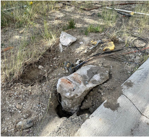
Figure 1 Location of old Jobbox, all cables ripped off.
