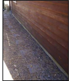
Un-maintained and dirty drip line treatment
